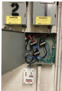
Figure 1 Surge protector installed at elevator splitter to ensure elevators are not affected by any electrical faults and to protect the elevator motors.
