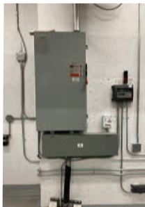
Figure 2 Surge Protector installed at chiller disconnect switch location. Device is currently up and running and is protecting the chiller from any electrical faults.
