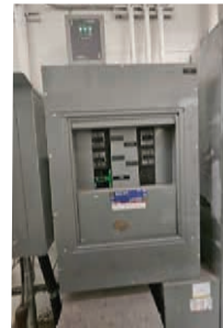
Figure 2 Surge protector installed at elevator panel location.
