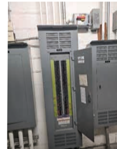
Figure 3 Surge protector installed at emergency lighting panel. External disconnect switch was used to accommodate the lack of space within panel.
